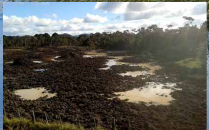
Elevated view of the constructed ephemeral wetland in the Wairua Oxbow. The ephemeral wetlands are one of the actions of the Wairua Oxbow Restoration Project, a collaboration between LW and Whangarei District Council.
